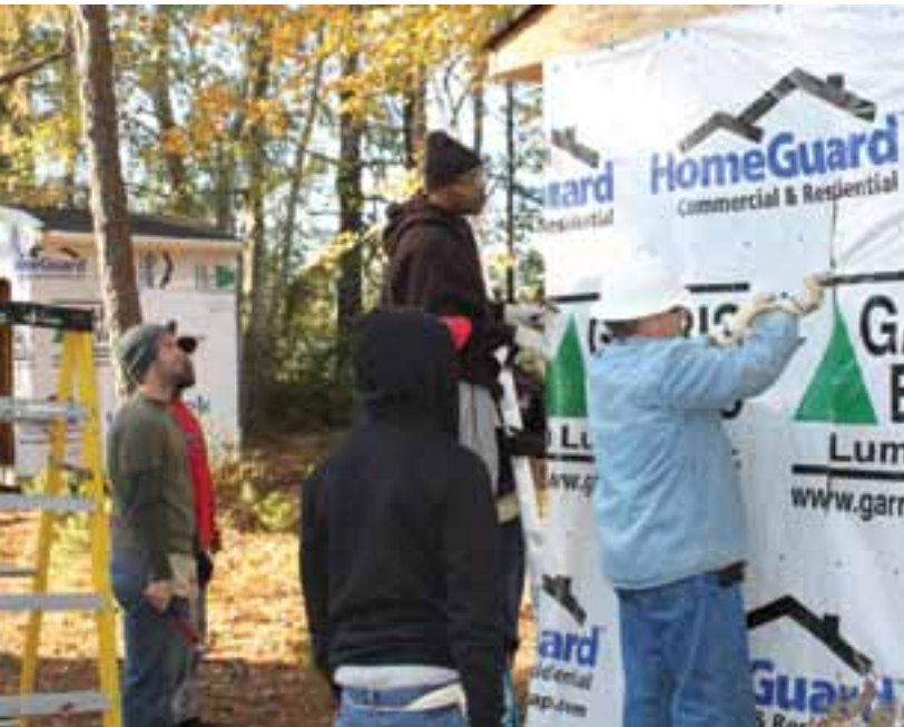
Students in Craven's Residential Green Building Trades/Weatherization Certificate program, top photo, take part in a Habitat for Humanity project in Havelock. In the bottom photo, instructor Keith Williams cuts through a thermal membrane for a doorway while a group of students looks on.
